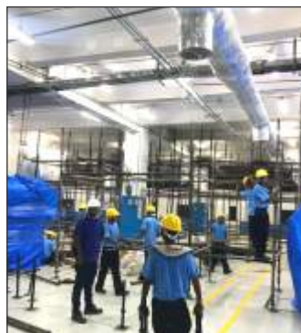
KELLOGGS INDIA LTD. Rehabilitation of Tank Deck Cost - 500 Lacs Location - Talaja, Mumbai
