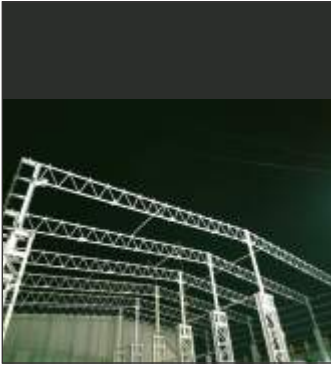
RELIABLE AUTOTECH PVT. LTD. Area: 25,000 Sq. Ft. Cost: 650 Lacs Consultant: Dandekar & Associates, Pune Location: Chakan, Pune
